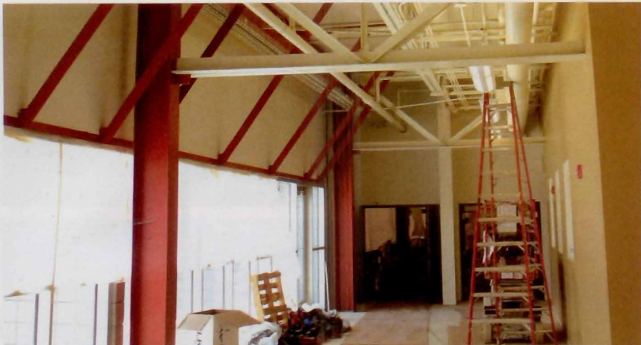
The $11.2 million school's interior leaves much of the structural and mechanical systems exposed, so students can observe how it was constructed. This meant the quality of workmanship had to be very high, even for normally hidden components.
