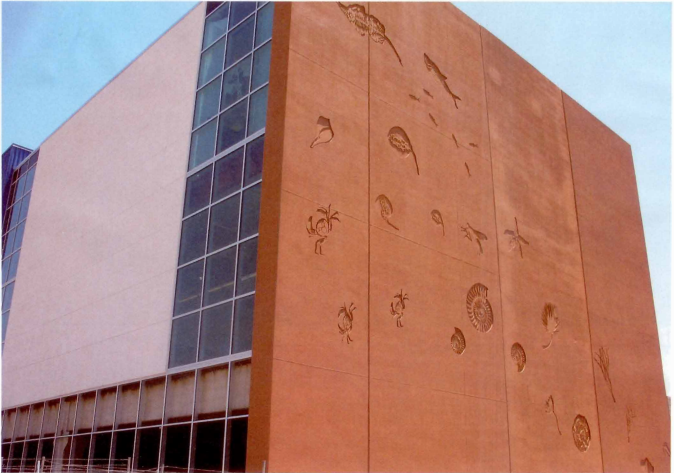
The Bioscience High School's massive tilt-up panels feature unique fossil shapes recessed into the concrete. The shapes depict single-cell organisms, invertebrates and mammals, showing the evolution of life on Earth. Photos by Scott Blair
