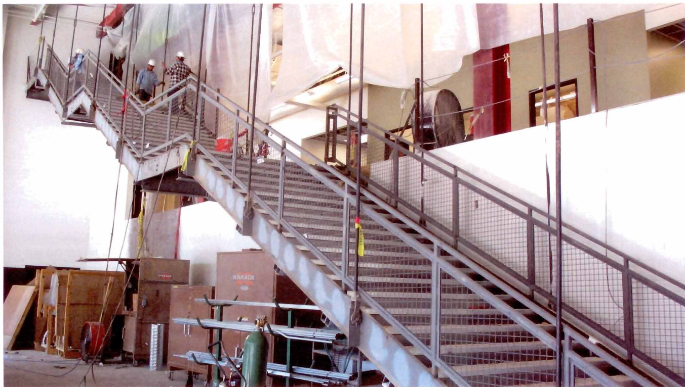
A massive metal stairway leads from the main assembly area up to the second and third floors. The stairs are suspended from the ceiling using long metal rods, clevis pins and turnbuckles which will eventually all be painted red.
